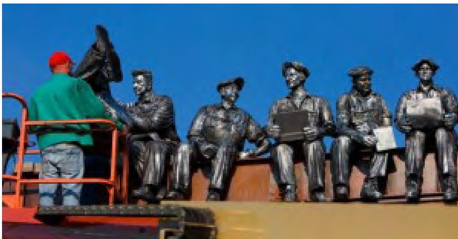
Artist Sergio Furnari, left, installs statues inspired by the 1932 photo "Lunchtime on Top of a Skyscraper" on top of the Industrial Revolution Eatery and Grille in Valparaiso. "(The restaurant's theme is) all about saluting America's greatness, a tribute to the people who build and protect this country," said owner Mike Leeson, of Schererville.
